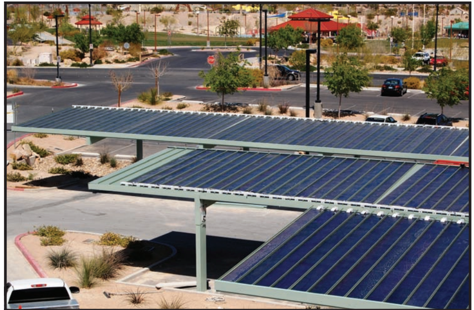
Solar covered parking at Centennial Hills Community Center
